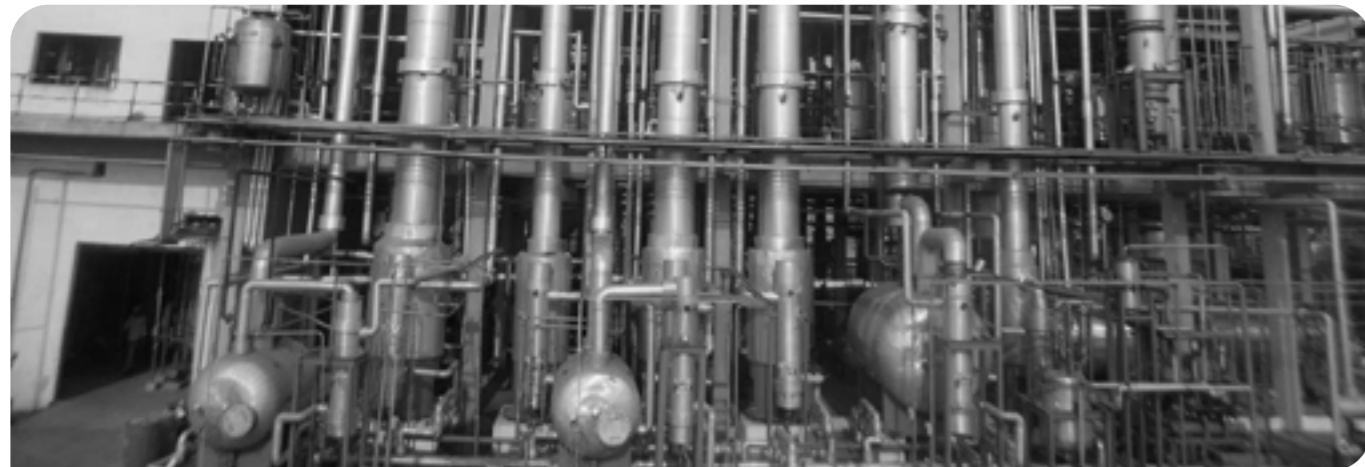
Solvent Recovery plant
