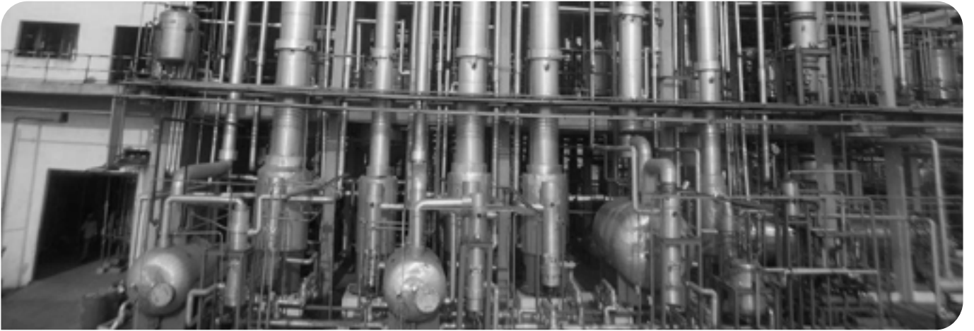
Solvent Recovery plant
